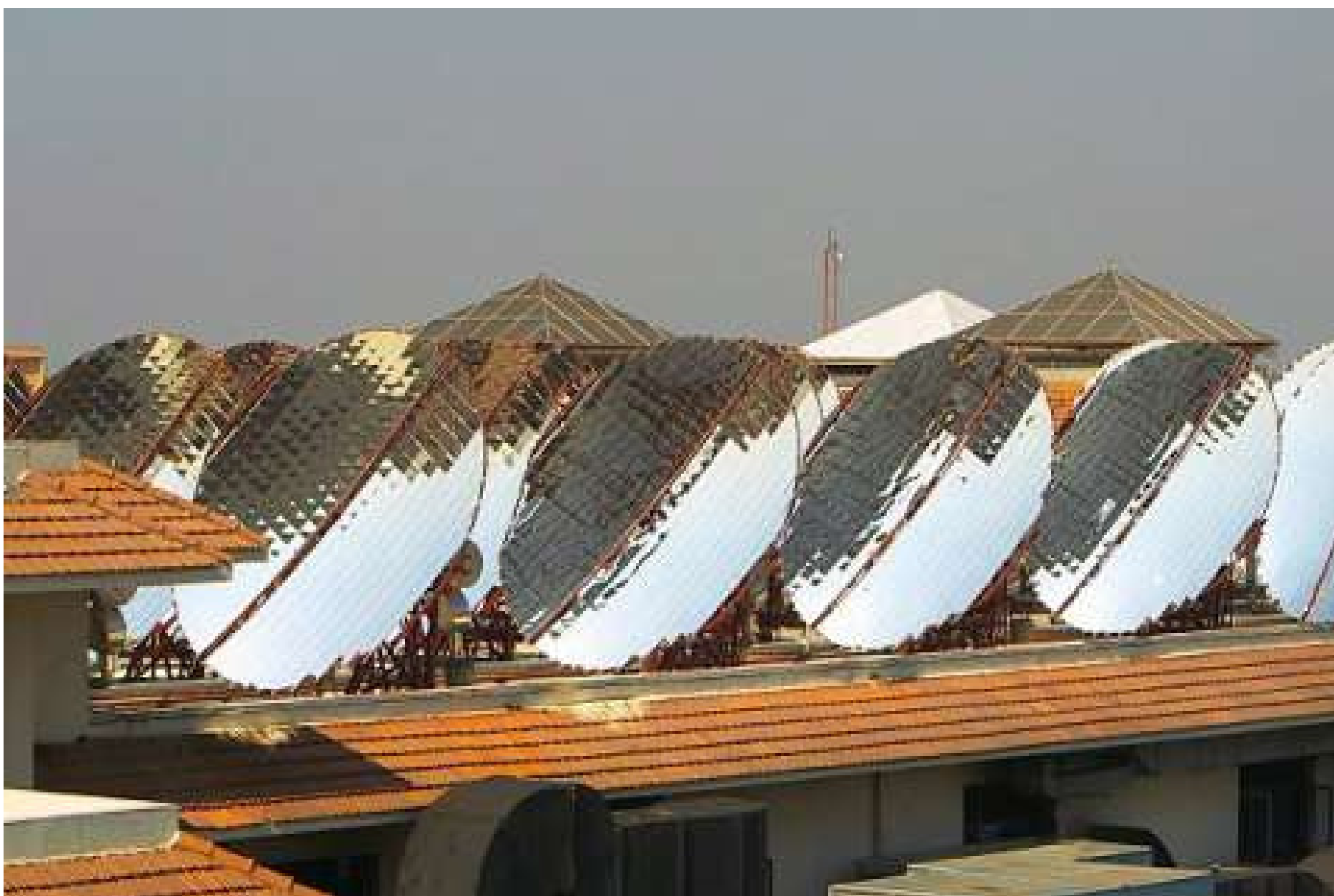
Solar panel on the roof of Shirdi Sai Temple.
